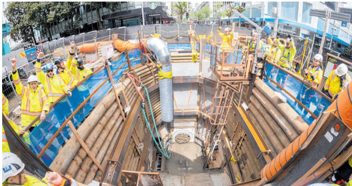
The micro tunnel borer breaks through at Victoria St East after laying a new wastewater pipe under Queen St.
